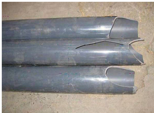
Damaged pipes inspected by CIS. DPRK Red Cross
