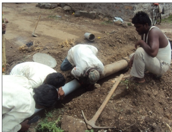
Villagers laying the pipeline to build up drainage system in the village. Photo: Indian Red Cross Society.
