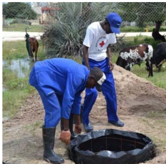
Namibia Red Cross Society volunteers erect a pit latrine Oshakati region of Namibia. SARO
