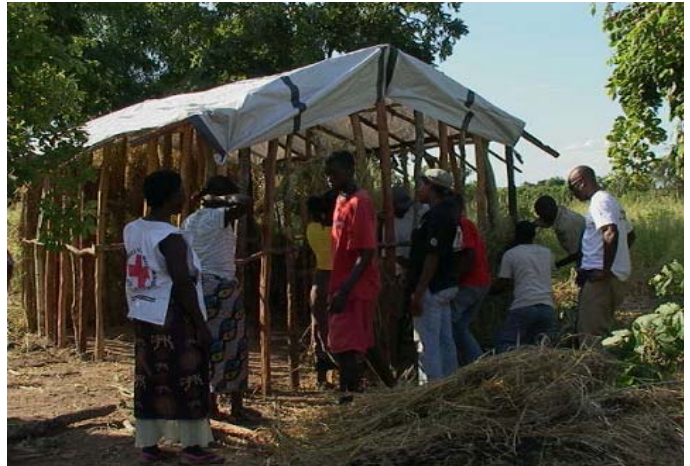
Shelter construction using shelter kit materials Limpopo valley in Gaza province 2011. Photo CVM
