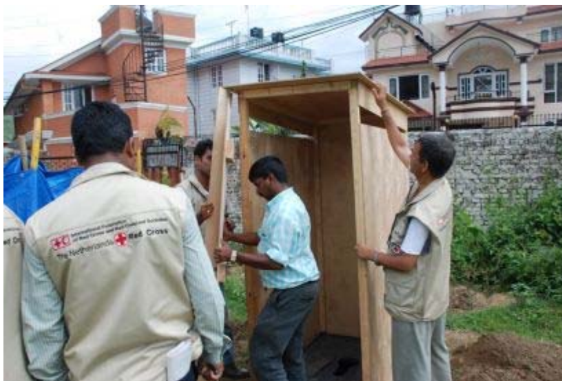
Participants installing a pit latrine during the water and sanitation training in Kathmandu. Photo: Nepal Red Cross Society.
