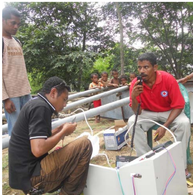
Early warning system equipment being set up in Buqui community under the community-based risk reduction (CBRR) project, Oecusse (Photo: CVTL)
