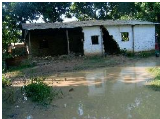
Impact of flooding: a destroyed house in Bangui district.
