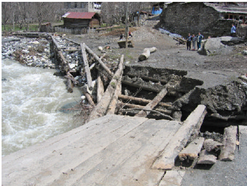
Cut off: floods caused damage to infrastructure, including this bridge in Ipari village, Upper Svaneti.
