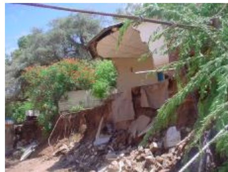
Hundreds of houses in Hargeisa were destroyed by the recent floods.
