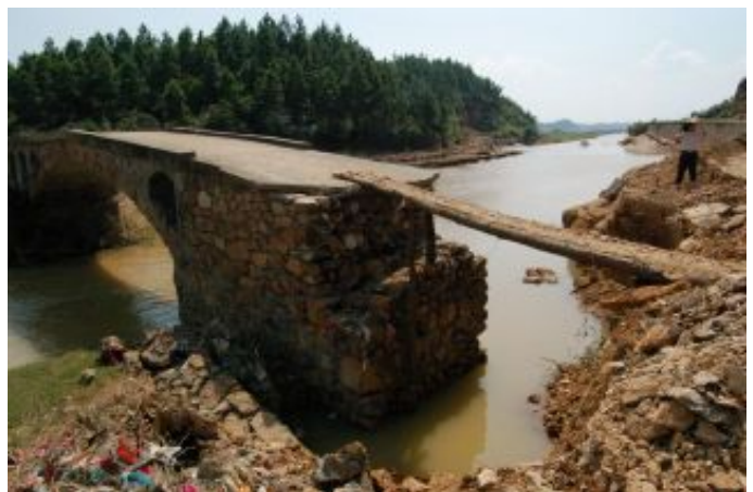
Floods have washed away bridges, impeding the daily lives of resident communities and challenging relief efforts.
