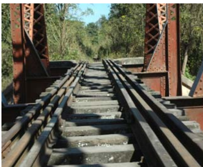
The railway bridge over Tartagal River was the only bridge left standing
