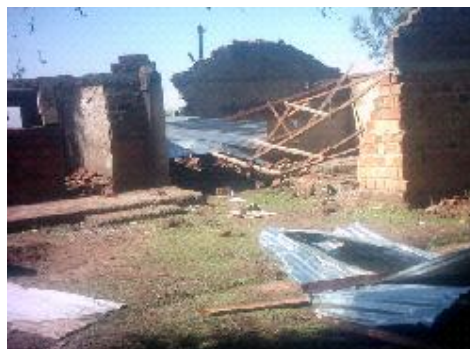
Photo above: One of the buildings totally destroyed during the storms.
