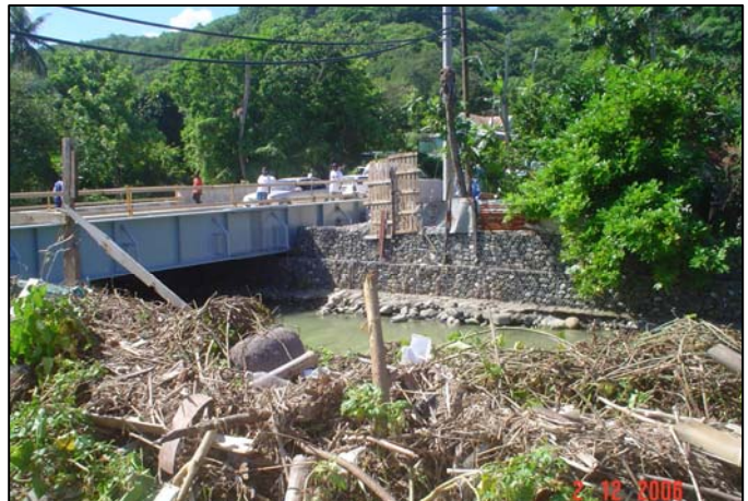
Debris and garbage were left behind by the floods. Source: International Federation
