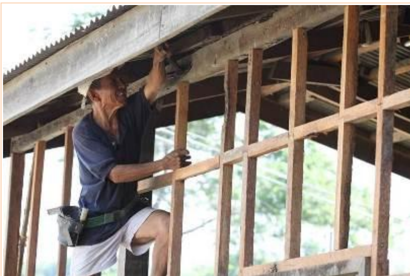
Peter Lacarte repairs the roof of his brother's house. His brother was one of the beneficiaries who received shelter repair kits from the Red Cross.
