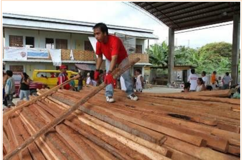
A member of the shelter project team checks the quality of lumber delivered by suppliers to ensure that it meets the standard.
