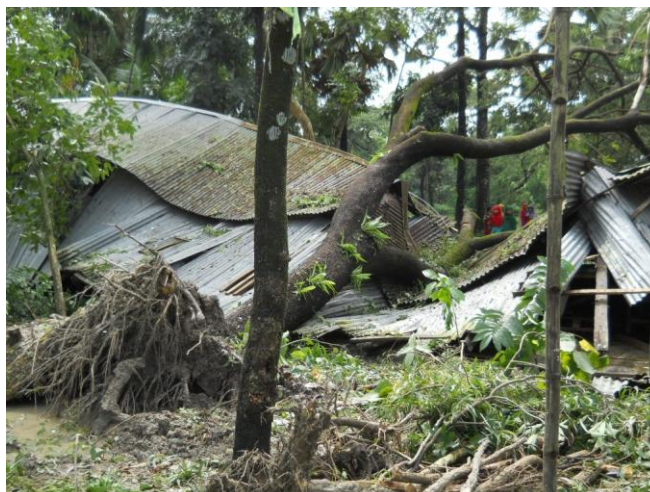
Uprooted trees causing hundreds of house damage in Hatiya Upazila of Noakhali district. Photo: BDRCS.
