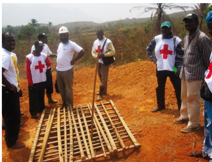
Construction of emergency latrines in Ngele and Pandu / Photo by Red Cross of DRC
