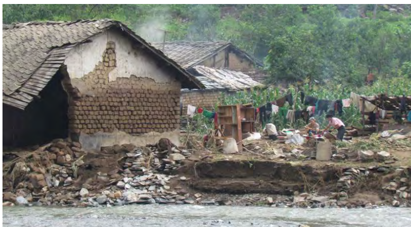
Torrential rains and subsequent floods damaged homes, infrastructure and livelihoods in DPRK. Affected families such as the one pictured above are living outside their damaged house in Ampo-ri community of Songchon county, South Phyongan Province. Photo: DPRK RCS
