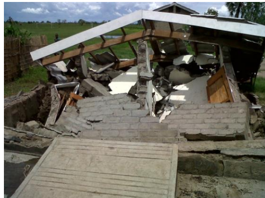
Even strong structures collapsed. A teachers house is badly damaged in Phalombe one of affected area/MRCS
