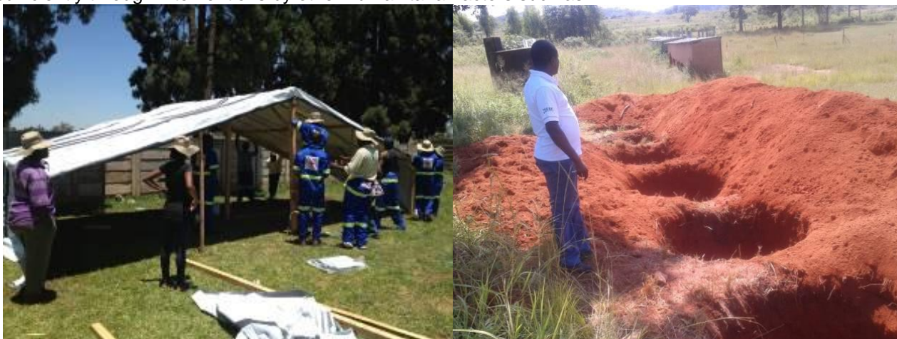
Left- Volunteers in practical training on emergency shelter construction; Right- excavated latrines pits in Zaka waiting construction. Photo: IFRC.
