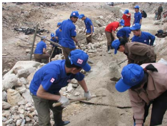
Community people actively participated in construction of stream embankment to reduce disaster risks in Dongyang-ri, Yangdok county, South Phyongan province. Photo: Kim Kwang Son, IFRC.
