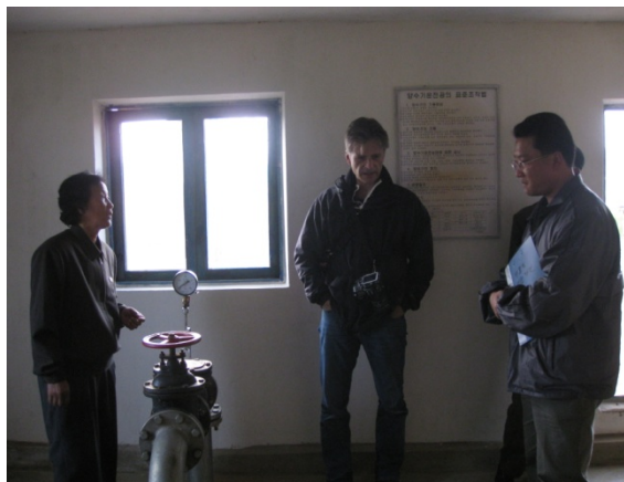
Handover and final monitoring for the constructed water supply system in Wonchonri, Taedong County on 12 October, 2011
