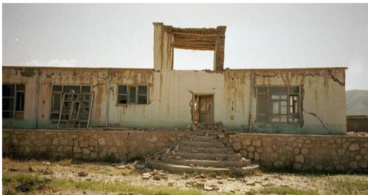
Even buildings which remained standing were not safe. Dangerous cracks were found on this.
