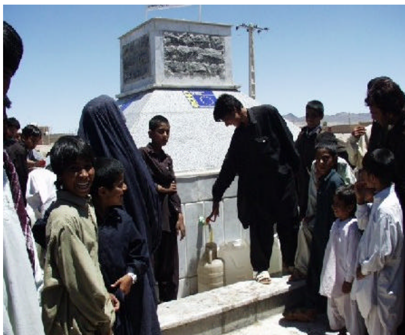
The construction of 4 public water distribution stations have provided the beneficiaries with permanent access to safe drinking water
