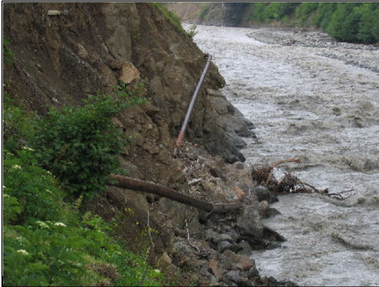
Water supply line cut in Oni: recent floods have destroyed the main water supply system in Oni, western Georgia. Red Cross will support the construction of a new system in the town to ensure its population have access to safe drinking water.
