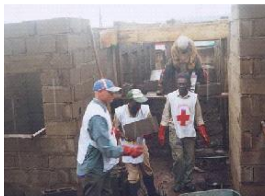
Red Cross volunteers participate in the construction of public latrines in Mbouda
