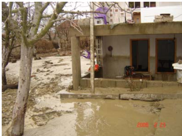
The flooding, caused by melting snow and heavy rains, caused damage to houses and personal belongings, agricultural land and equipment, and the power system
