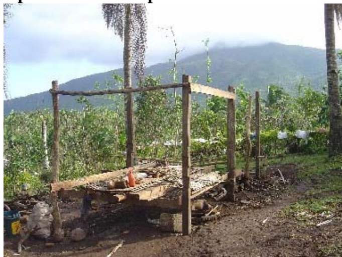
This is the sad remnant of one home that housed a family of nine
