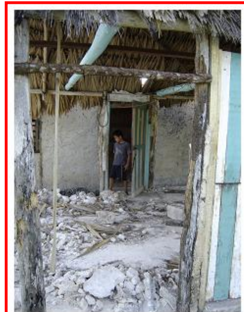
Destroyed house in Belize after Hurricane Dean's passage.
