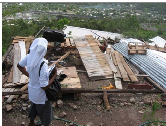
House completely destroyed by Hurricane Dean Source: International Federation
