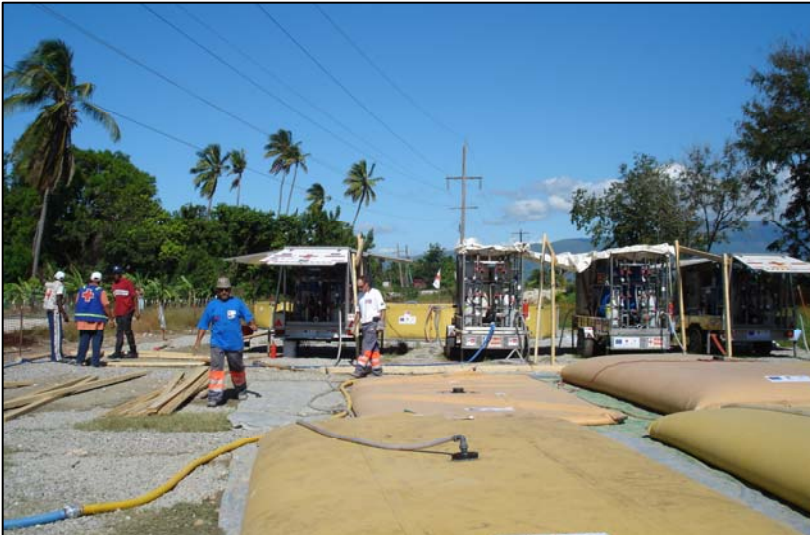
Bladder tanks installed in the Dominican Republic. Source: International Federation
