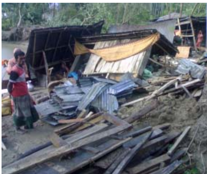
Destroyed houses in Bhola.
