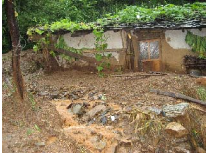
A house in Koksan that has been completely destroyed by floods. DPRK Red Cross.
