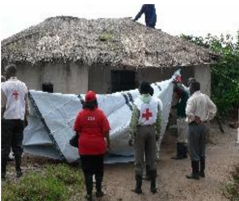
ZRCS action team covering a dwelling with tarpaulin in Kizhingezhinge, Solwezi to prevent it from further damage
