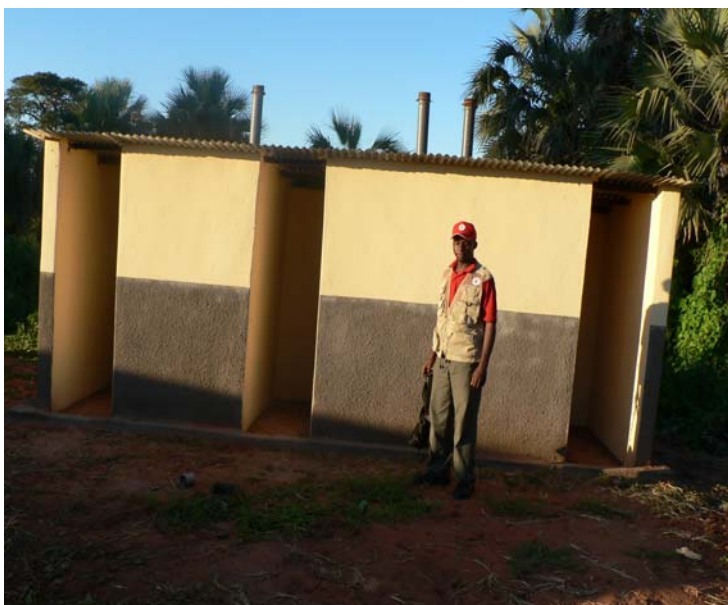
Completed VIP latrines at Katondwe School in Luangwa District ( Zambia Red Cross )
