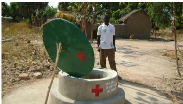
This water well was improved and treated by Chad Red Cross volunteers.
