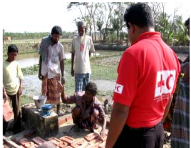
Under Red Cross Red Crescent programme framework; a tube well is being repaired in the district of Patuakhali with the assistance of the community people.
