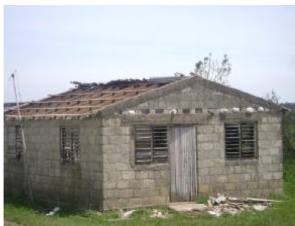
A damaged roof top in the municipality of La Palma. Source: International Federation
