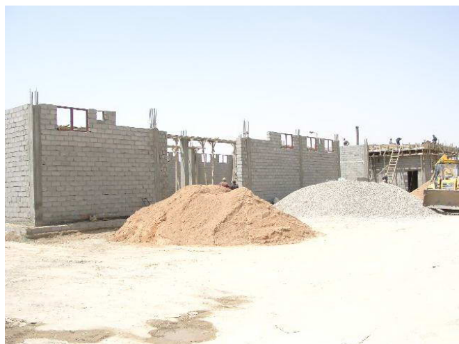
Baghdad regional warehouse and cold store construction project will be continued throughout 2009 and is expected to be completed in September 2009.
