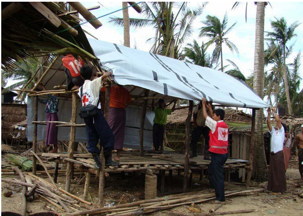
Rebuilding efforts underway in Bogale with the support of local Myanmar Red Cross Society volunteers.
