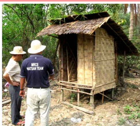
Strong community participation has contributed to the success of latrine construction projects. (Photo: Myanmar Red Cross Society)
