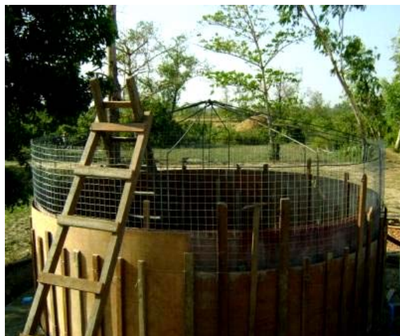
A Ferro cement tank under construction in Mawlamyinegyun. (Photo: Myanmar Red Cross Society)
