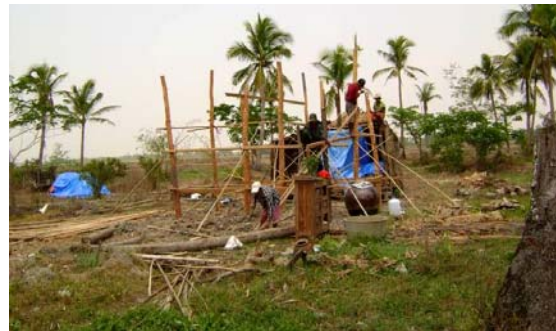
A woman ( top picture ) weaves palm leaves for the roof of her new house ( bottom picture ) as her children look. The house is being built by her husband, U Chitto, with the help of three local labourers, as part of a pilot scheme for the household shelter programme. The family was one of five households in Thet Kel Seike village in Bogale, selected to participate in the scheme. Timber from their damaged home was salvaged and used to build the new one. (Photo: International Federation/Patrick Elliott)
