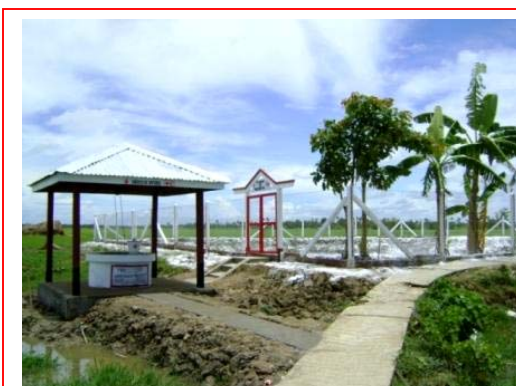
A rehabilitated pond and a new tube well in Ywar Ma village in Mawlamyinegyun township. The water supplied to the well is cleaned and made safe for drinking through a sand filter. (Photo: MRCS)
