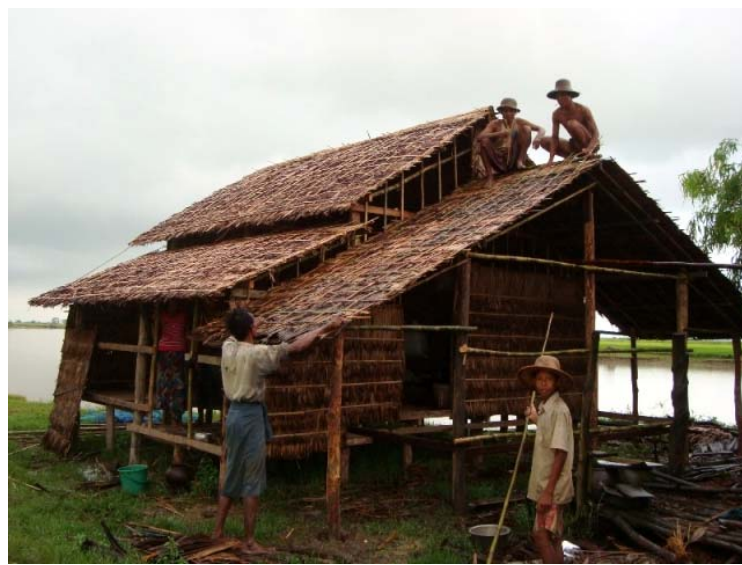
The household shelter project targeted for 8,000 households has been well received by vulnerable communities. A second phase of constructions for 7,000 households is targeted to begin in February. This photograph features a shelter being constructed in Swe Sone village in Labutta township. (Photo: Ye Thaug Htut / IFRC)
