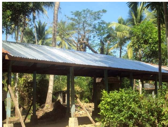
The Repairs to Damaged Community Buildings and Infrastructure project, is community-driven and has been well received by targeted communities across 11 townships. A second phase is planned for March. This photo features a repaired roof of the entryway to a monastery in Nyaung Wyne Gyi village in Maubin township. (Photo: Myanmar Red Cross Society)
