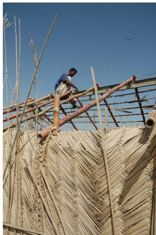
Shelter materials supplied in 2007 are being recycled for more durable construction in 2008. This man in Tanzag village, near Turbat (Baluchistan) is utilising tools and bamboo supplied by the PRCS/ Federation. The locally-available date palm matting is a popular wall/roofing material. (Photo: Mubashir Fida, IFRC).
