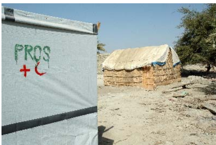
A latrine installed by the PRCS in Turbat. The 'pull-flush' design has proved to be more durable and acceptable to communities than pit latrines. The PRCS latrines installed in 2007 are still being used in 2008. (Photo: Mubashir Fida, IFRC)
