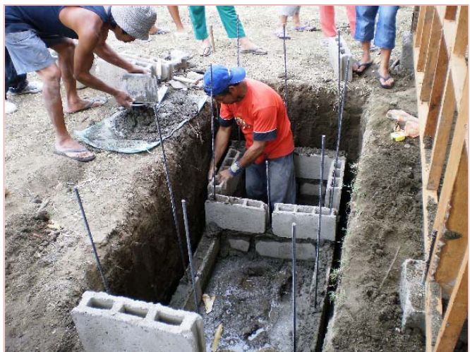
Construction of a septic tank for the pour-flush latrine. A latrine is planned for each transitional shelter. Photo: IFRC
