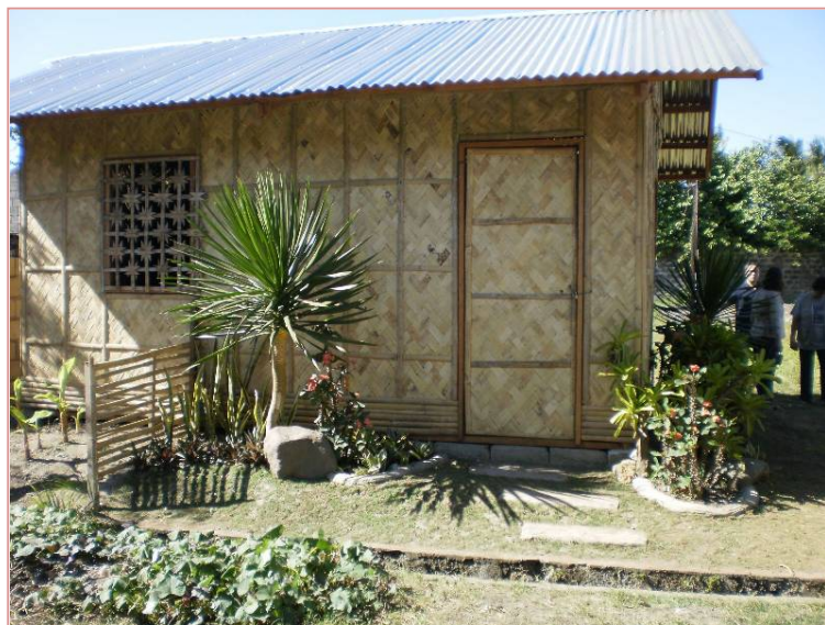
Construction of model houses – with latrines and septic tanks – has been completed in Laguna. (Photo: Alexander Mikadze, IFRC)
