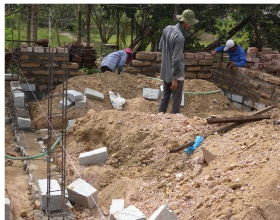
A beneficiary family's house under construction in Duc Phu commune, Mo Duc district, Quang Ngai province: up to 650 houses across seven provinces are expected to be completed by the end of September 2010. (Photo: DWF)
