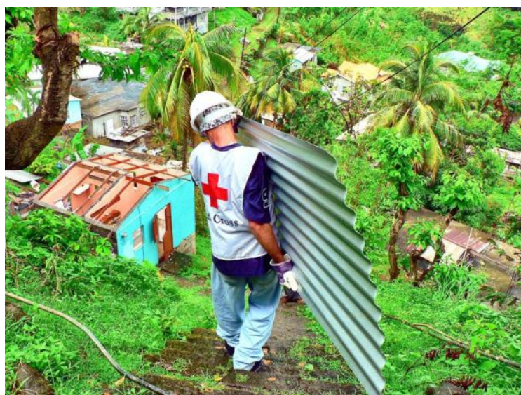
The National Societies of Barbados and Saint Vincent and the Grenadines are working to provide safer roofs to the affected families. Source: SVGRC.
