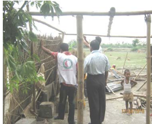
BDRCS volunteers assisting people to fix damaged houses, in Velacopa village, Kurigram Photo credit: BDRCS/IFRC
