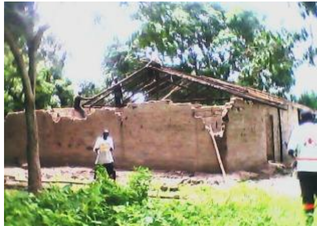
This house, like many others, was destroyed by the torrential rains.
