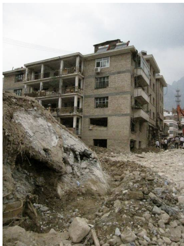
One of the buildings destroyed in the mudslide triggered by floods on 8 August in Zhouqu, Gansu province. Photo: RCSC
