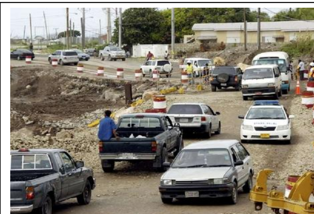
Heavy rains caused Hope River to wash away the ford which links to Harbour View to Bull Bay. Source: The Gleaner / Norman Grindley.
